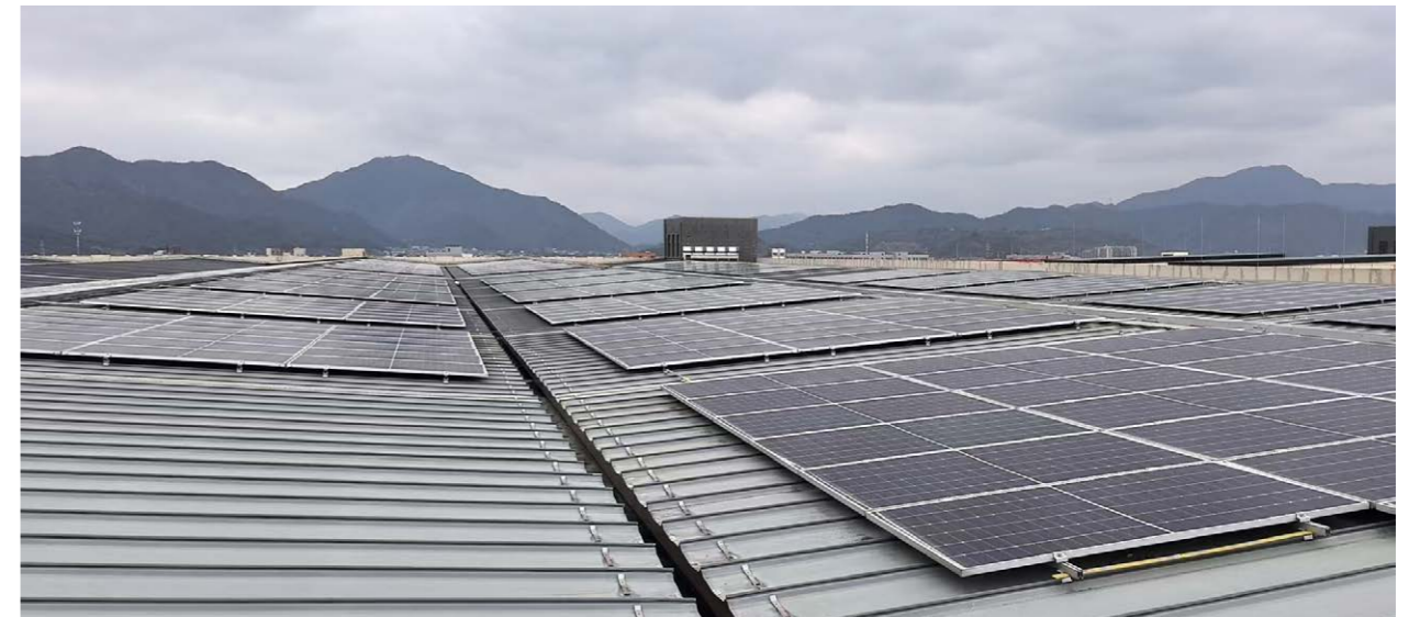
PV Solar Power Generation Installation in Xiangshan Logistics Warehouse
